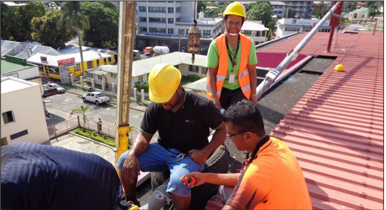
Geospatial Information System (GIS) Unit while installing the new Global Navigation Satellite System at the Head Office in Suva
