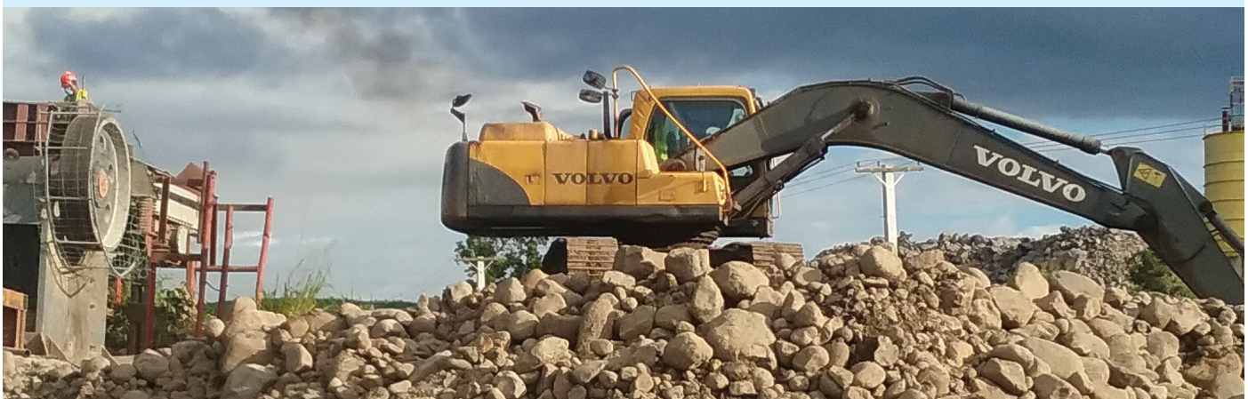
Mataqali Matarisiga of the Yavusa Tunuloa in Vitogo, Lautoka runs a competitive business as Petra Industries that deals from crushing of stones/rocks to producing concrete and cement
